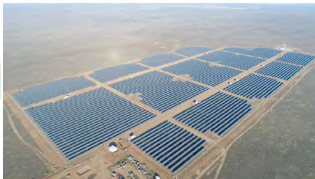
Maloderbetovskaya Solar Facility, Kalmyk Republic
